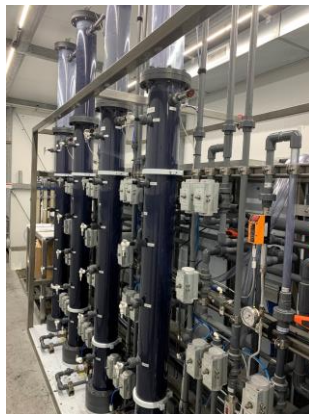
BAC and GAC Filter Pilot Unit (Intuitech)
