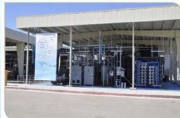
The Water Purification Demonstration Project is evaluating the feasibility of indirect potable reuse/reservoir augmentation.
